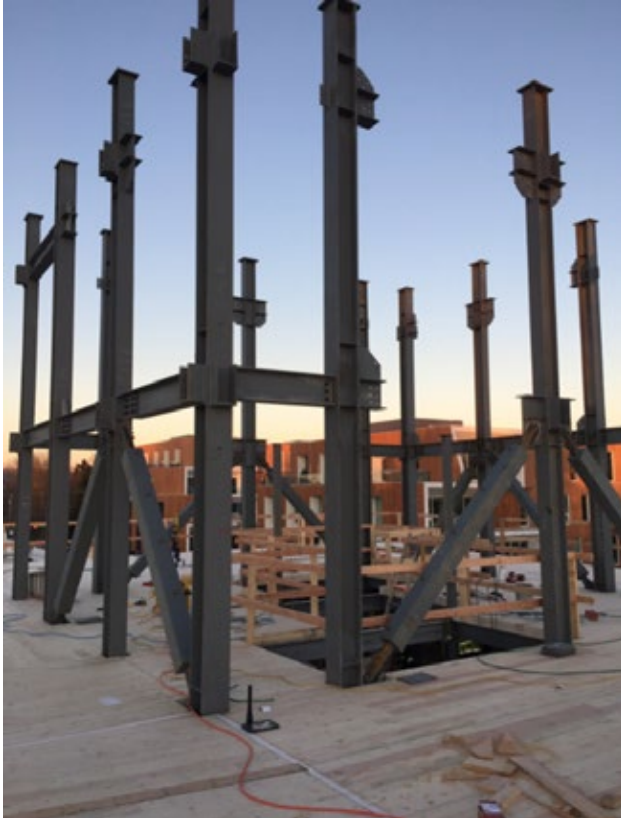
FIGURE 5.17: CLT POST AND BEAM STRUCTURE WITH BUCKLING RESTRAINED BRACED FRAME CORE Carbon 12, Portland, OR; Source: Kaiser+Path
