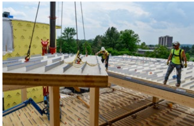
TOP – FIGURE 5.11: COMPOSITE CONCRETE-TIMBER SLAB WITH ACOUSTIC MAT AND INCLINED SCREW REINFORCING
