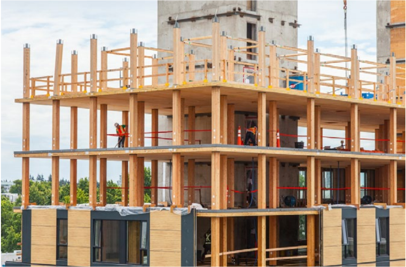
FIGURE 6.6: PREFABRICATED FACADE PANELS FOLLOW CLOSELY BEHIND STRUCTURAL FRAMING Brock Commons, University of British Columbia; Source: Ralph Austin at Seagate Structures
