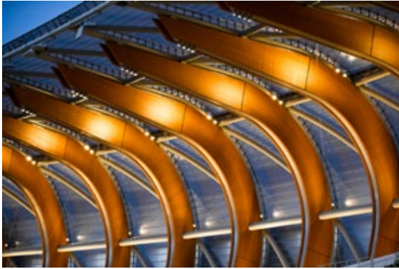
OVER 462 DOUGLAS FIR GLULAM STRUCTURAL WOOD PIECES WERE USED TO CREATE 77 UNIQUE CURVES, EACH CONTAINING SIX PIECES OF BENT WOOD. Photo Credit: Matt Parker/UO Track and Field
