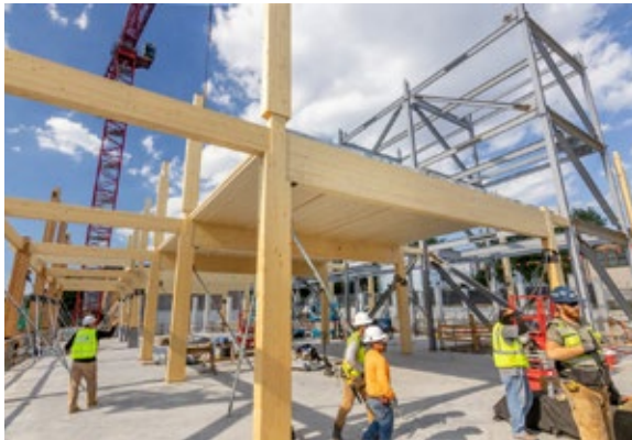
FIGURE 2: THE STEEL CORE ACTS AS THE LATERAL BRACING SYSTEM, SAVING SIGNIFICANT CONSTRUCTION TIME COMPARED TO A TRADITIONAL CONCRETE OR CMU CORE.
