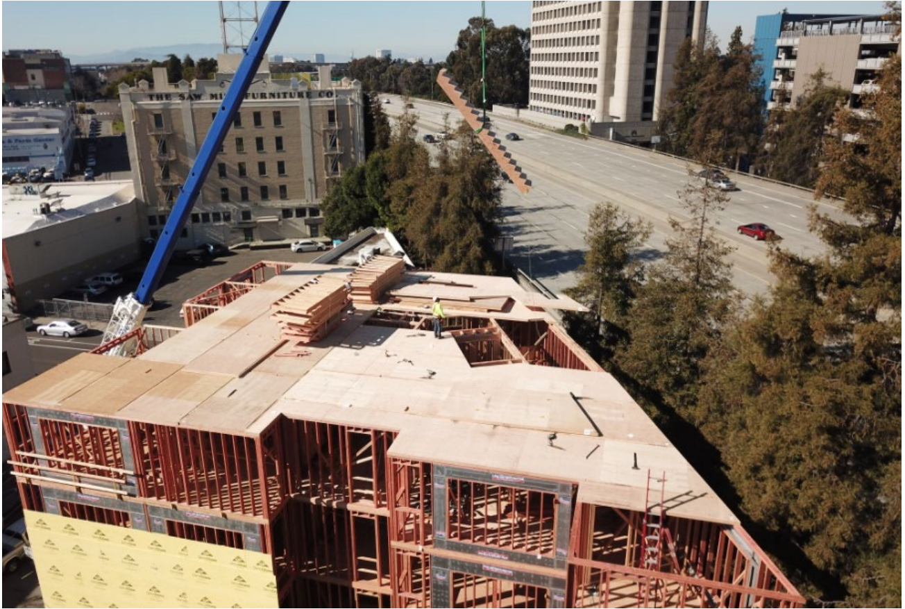
FIGURE 6.5: PRECISION COMPONENTS QUICKLY ASSEMBLED ON A CONSTRAINED SITE Project One, San Francisco, California, Gurnet Point Construction, DCI Engineers, Freres Lumber Co.
