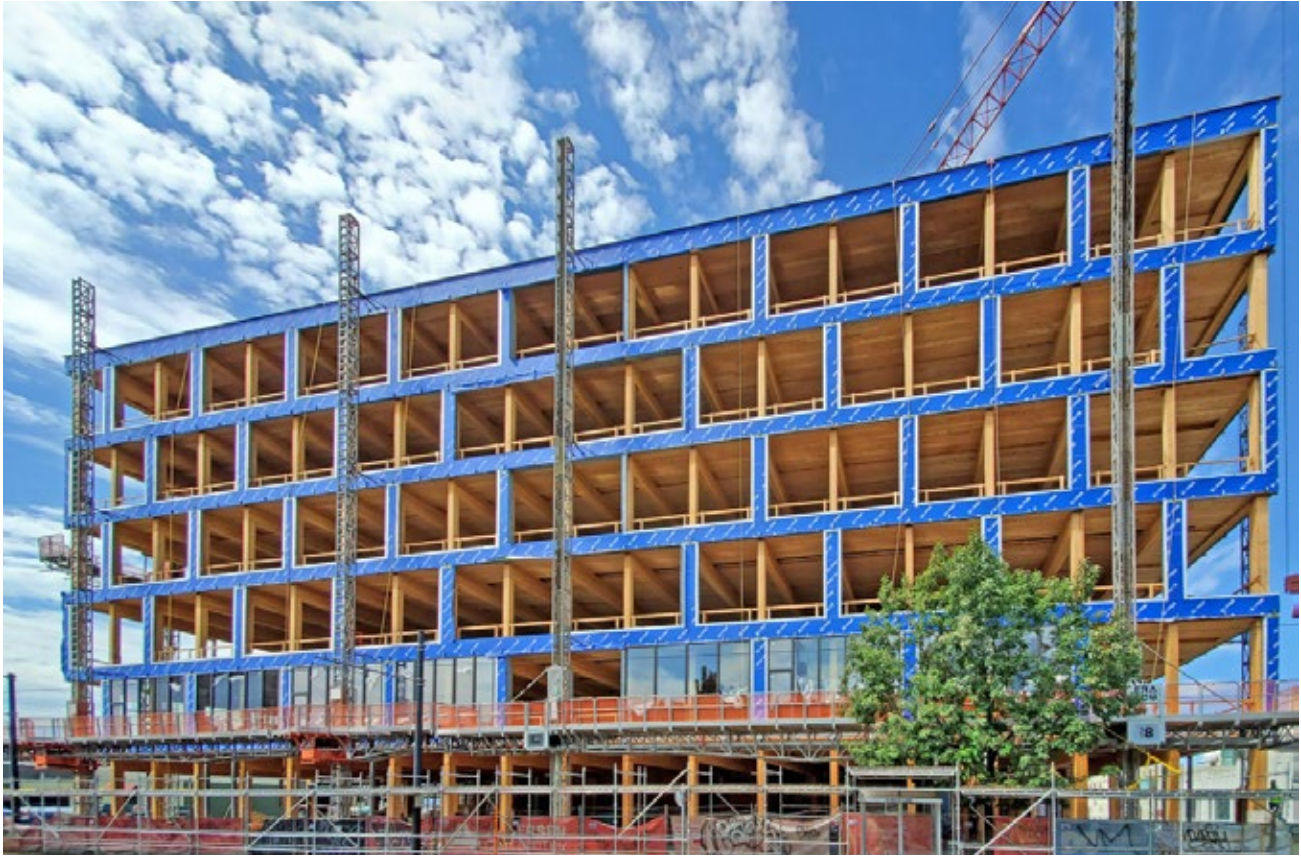
FIGURE 6.19: DISTRICT OFFICE IMPLEMENTED A MOISTURE MANAGEMENT PLAN
